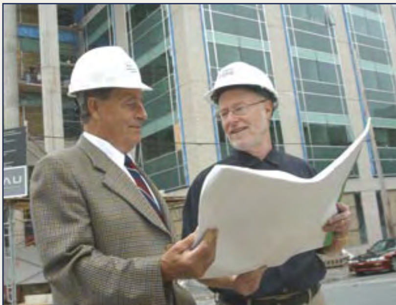
Ken Rowe and President Tom Travis visit the project during the construction phase
